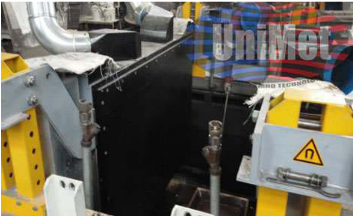
Fig. 3. LHMS inductors on the casting pit
