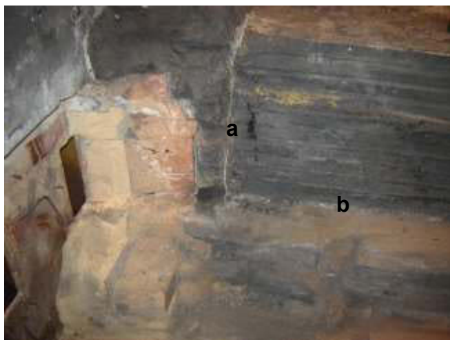
Fig. 10. Leakage of metal (a) at perimeter seam. Metal leaked from collector bar and also ran under the cathode blocks (b)
