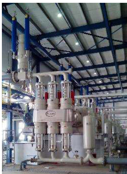
Fig. 1. Seven sets of double hose-diaphragm pumps
