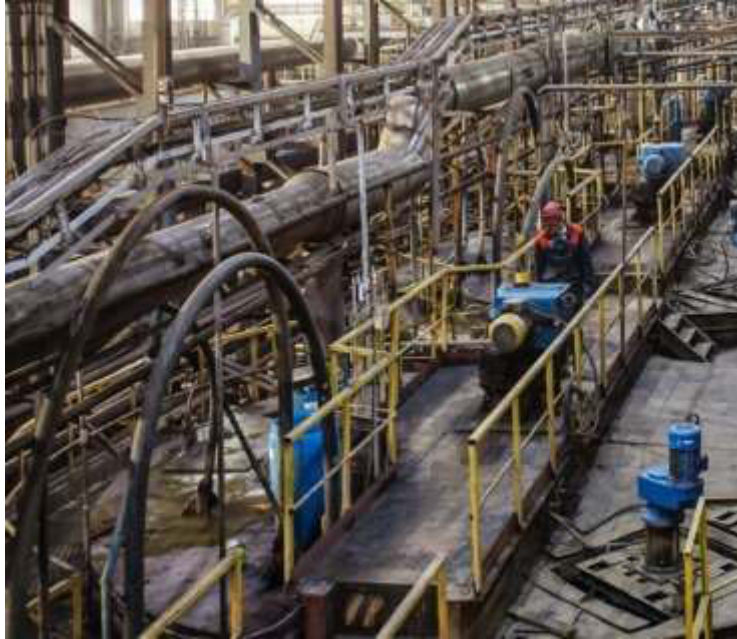
Fig. 2. Proper implementation of the process of moving activated coal through the sorption process.
