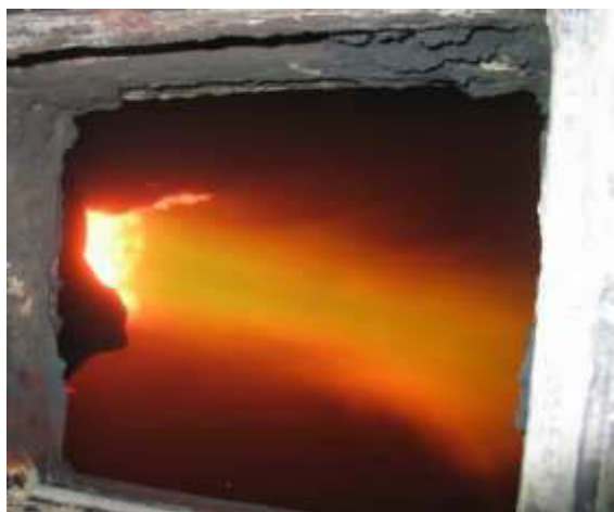
Fig. 3. Uptake shaft - waste heat boiler junction, December 2016 (from the WHB inspection window)
